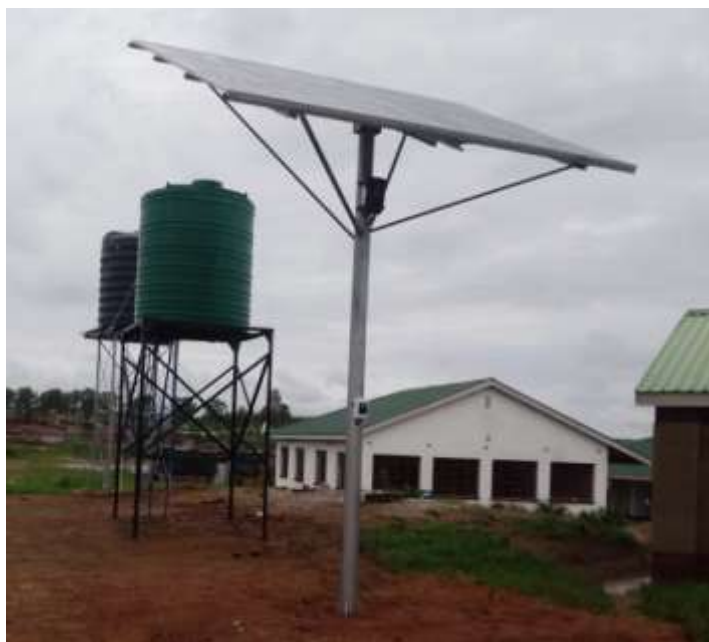
Figure 8: The Installation at St Catherine of Alexandria School
